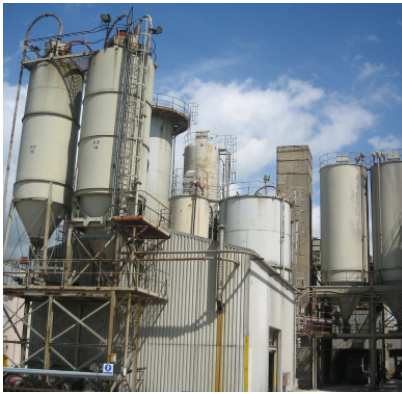
An example of silo level measurement.
