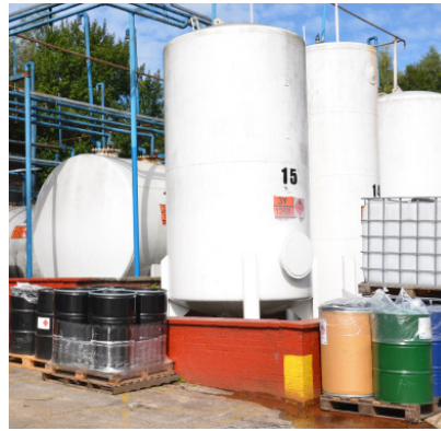
An example of tank level measurement.
