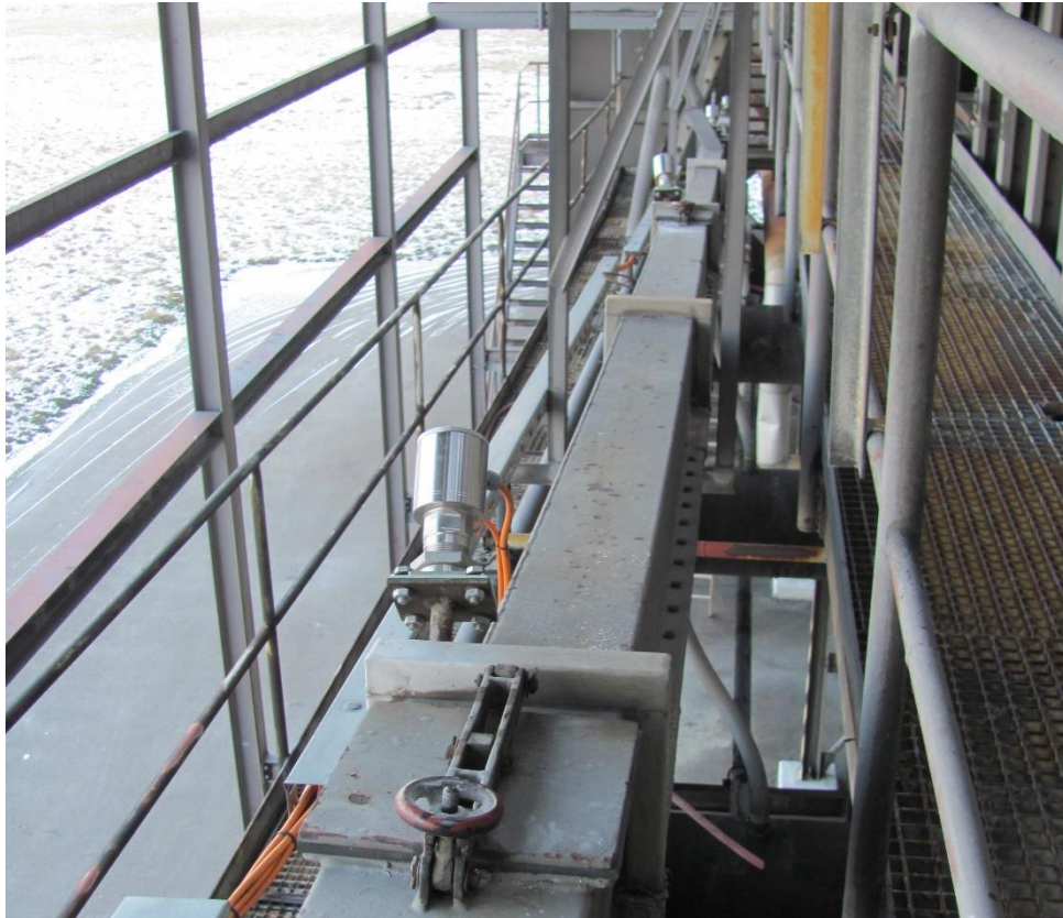
FS 510 installed on the conveyor belt for the aluminum oxide
